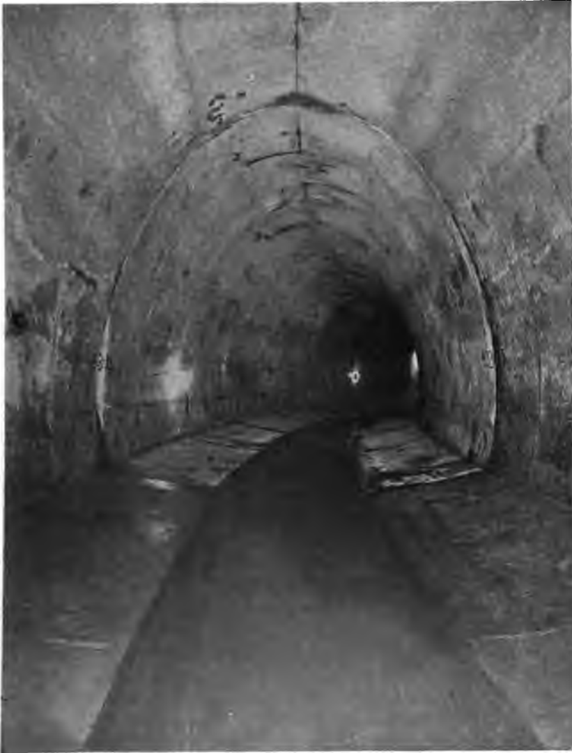
PLATE 75.—Contract 11. Cut-and-cover Aqueduct on Curve. Arch cast with aid of steel forms built wedge-shaped in 5-foot lengths to 200 feet radius. Section 17 feet high by 17 feet 6 inches wide.
